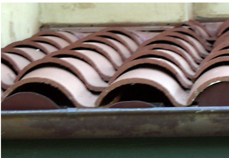
Figure 9. Two of the three visible bird stops shown in this clay barrel tile roof covering have been improperly installed or have become detached. Inspection of these should be part of a regular (annual) inspection and repair plan. Photo: Stephen L. Quarles.
