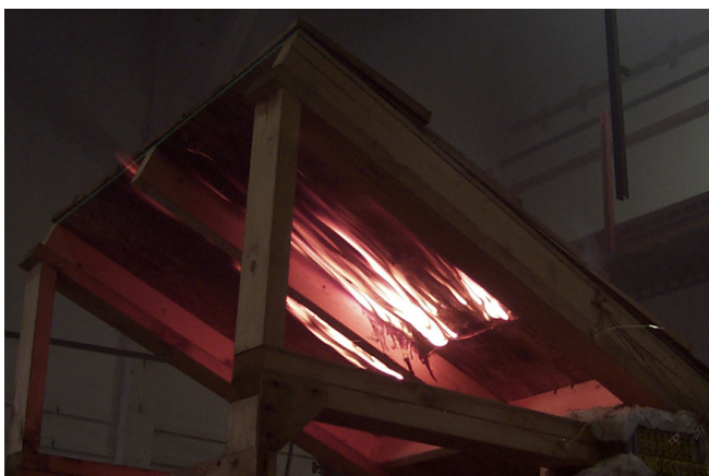
Figure 3. Demonstration of a flame-through (burn-through), passing from the roof covering to the underside of the roof deck. As constructed, this is not a Class A roof covering because it allowed flame penetration when subjected to a Class A burning brand. Photo: Stephen L. Quarles.
