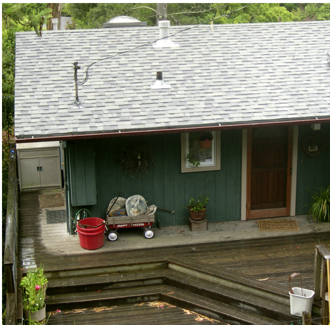
Figure 12. The wide overhang on this home protects the exterior wall from rain. Since many water-related problems in buildings can be traced to leaks at penetrations in the exterior wall (e.g., at windows and doors), limiting exposure would reduce the occurrence of water-related problems. Photo: Stephen L. Quarles.
